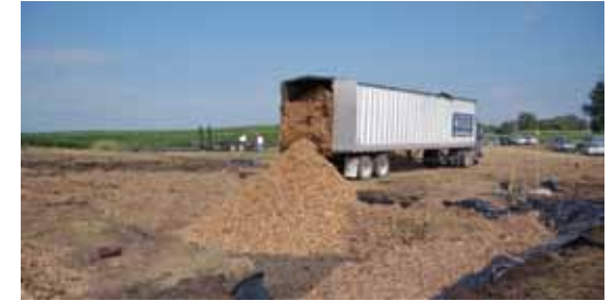
Microorganisms colonize the wood chips and use them as a food source, while breaking down the nitrate in the water, and expelling it as a gas.
