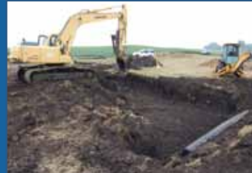
◀ This view looks from southeast to northwest with upslope generally from right to left. Both control structures are visible and excavation has now started on the processing section of the bioreactor. The processing section of this bioreactor site measures 25 feet by 50 feet, making it the largest known tile line bioreactor in the U.S.
