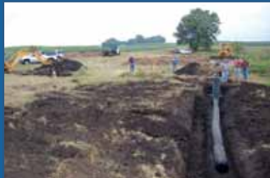
◀ This photo looks from south to north and upslope is from right-to-left. The lower control structure is in place at the right, with a tile line installed to collect the bioreactor output (extending into the bottom of the photo). Excavation is beginning for placement of the upper control structure at the left by the backhoe.
